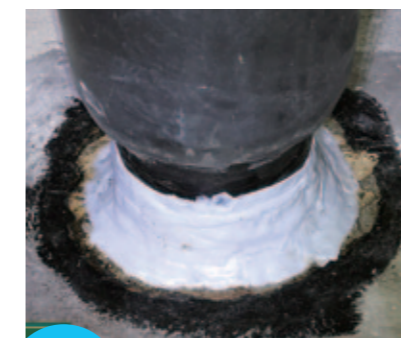
止水 Water stop パイプ貫通孔の止水 Water stop for pipe perforation holes
