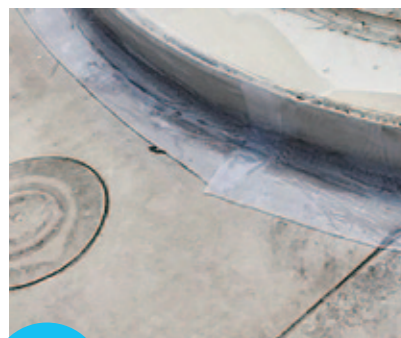
止水 Water stop 屋上防水の漏水補修 Waterproof roof water leakage repair
