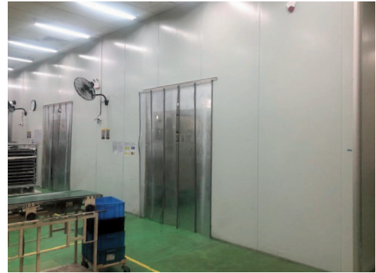
Partitioning the equipment and adding flame retardant vinyl curtains at the entrance and exit
