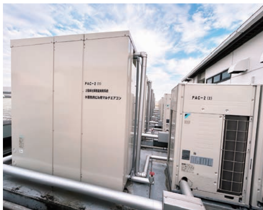
Air conditioning system equipped with an ice thermal storage tank
